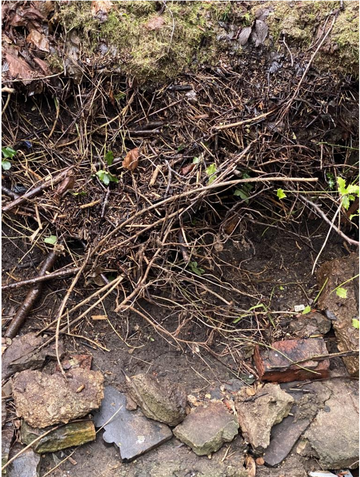
Remnants of a bank retaining wall washed away on 26 December 2020.
