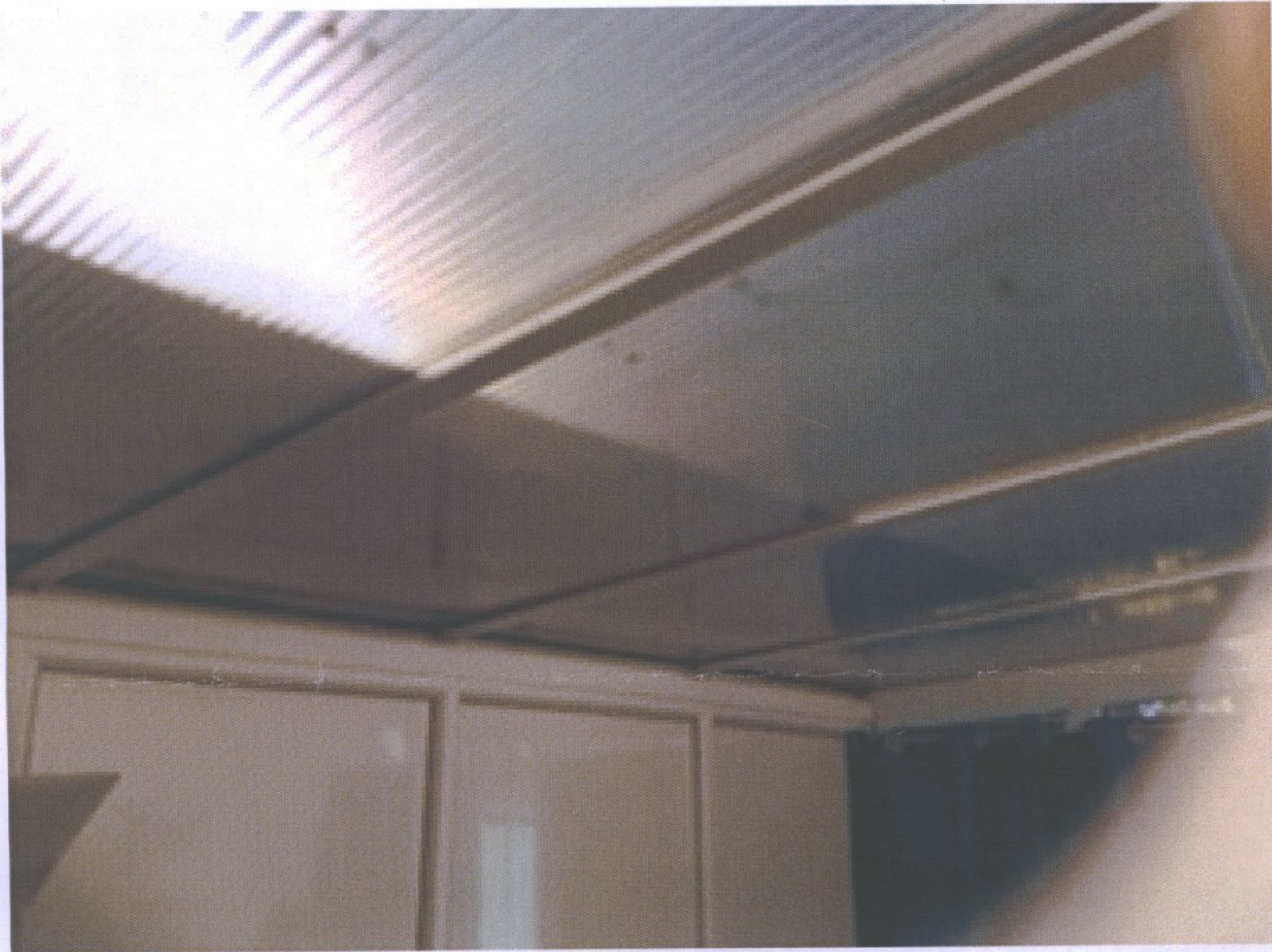
Photo taken mid afternoon in August when sun high in the sky showing shadow covering one third of the conservatory at no 34 Noverton Lane.
