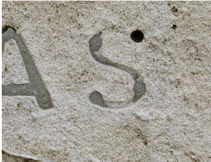
Fig 38: detail of mortar fill missing from incision
