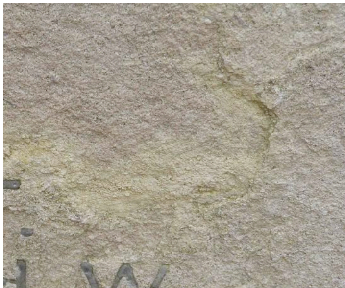
Fig 13: stonework on east side panel showing deterioration through clay swelling
