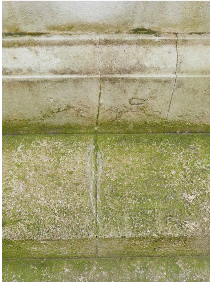
Fig 9: crack in moulded base plinth stone immediately above joint in step
