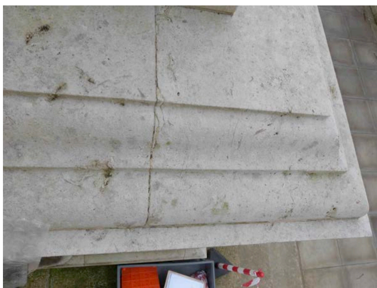
Fig 34: detail of moulding showing cracked joints
