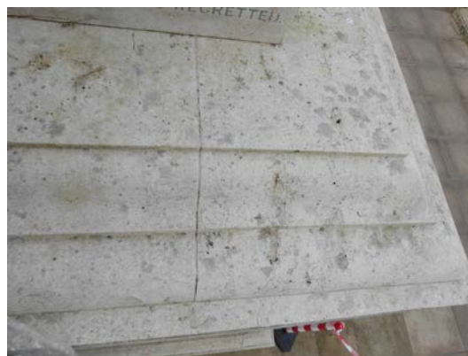
Fig 24: erosion of sky face of moulding
