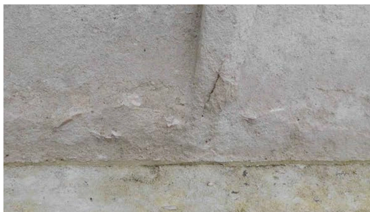
Fig 28: detail of deterioration at tip of sword
