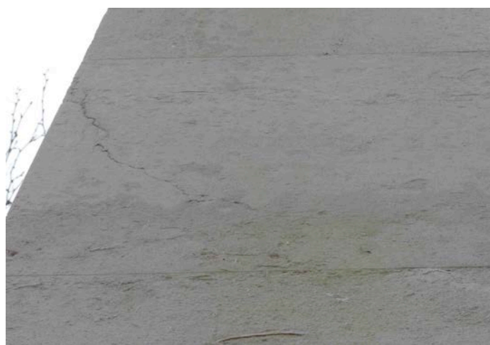
Fig 31: natural fault in obelisk stone
