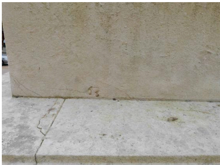
Fig 35: detail of moulding and obelisk plinth showing cracks in stone
