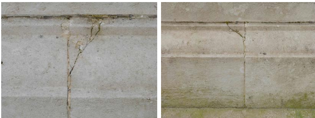
Fig 10 and 11: spalling of base plinth stone due to corrosion of cramps (south and north elevations)
