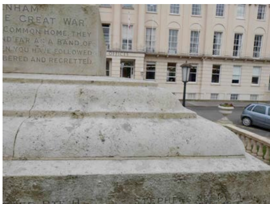
Fig 23: cracked pointing at base of moulding
