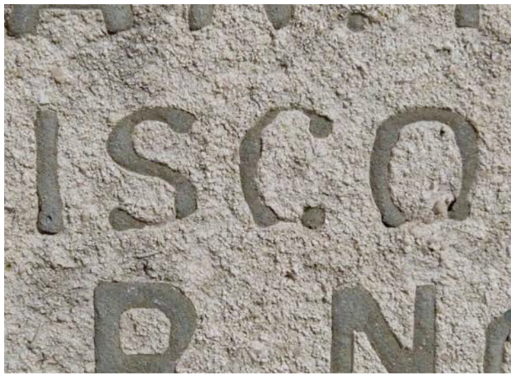
Fig 39: detail showing erosion of both incision and mortar fill
