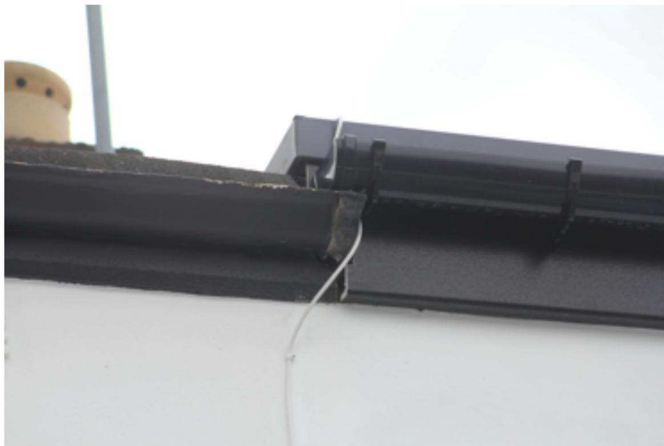
Figure 3: Changes to guttering between two properties
