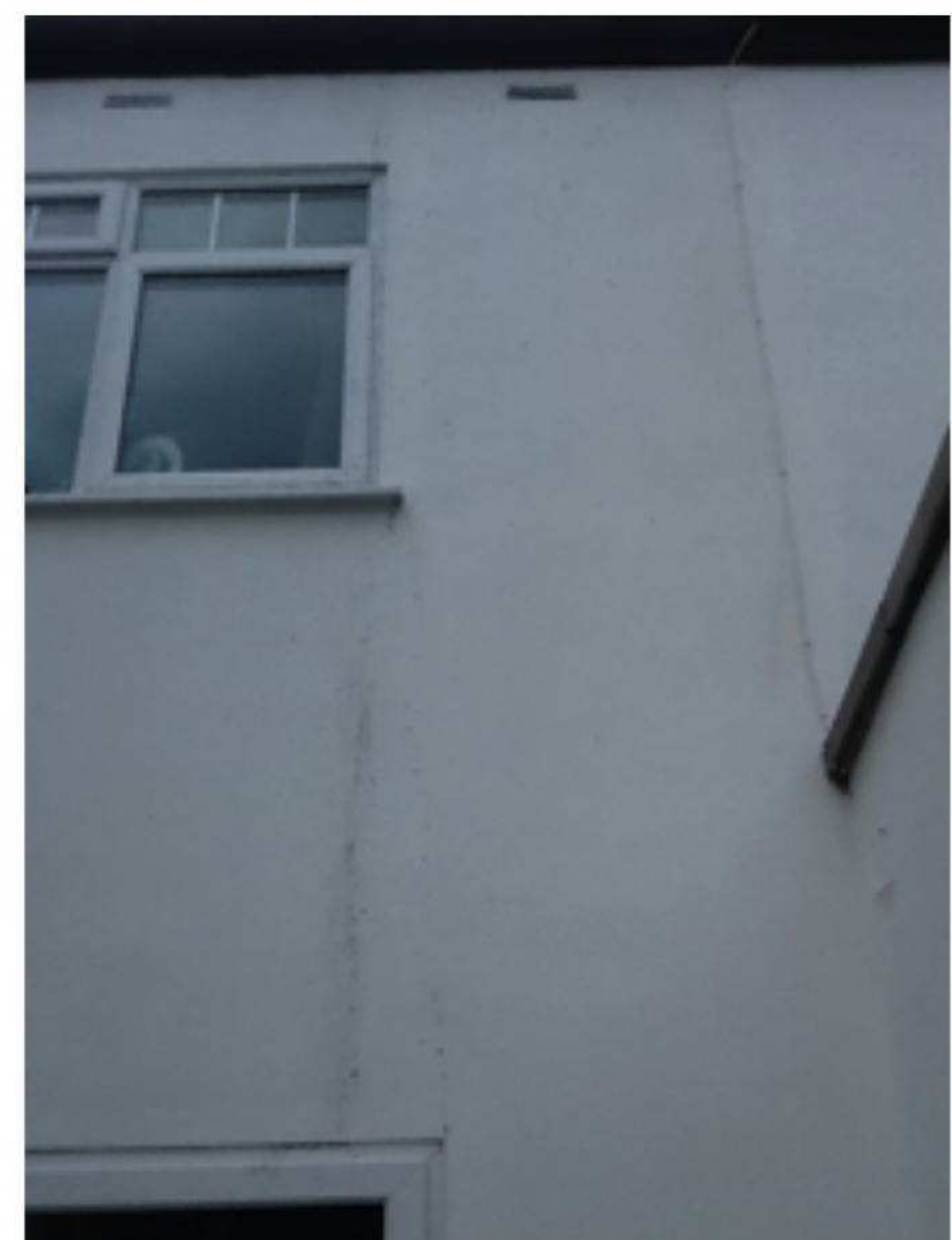
Figure 4: Dirt from guttering on wall
