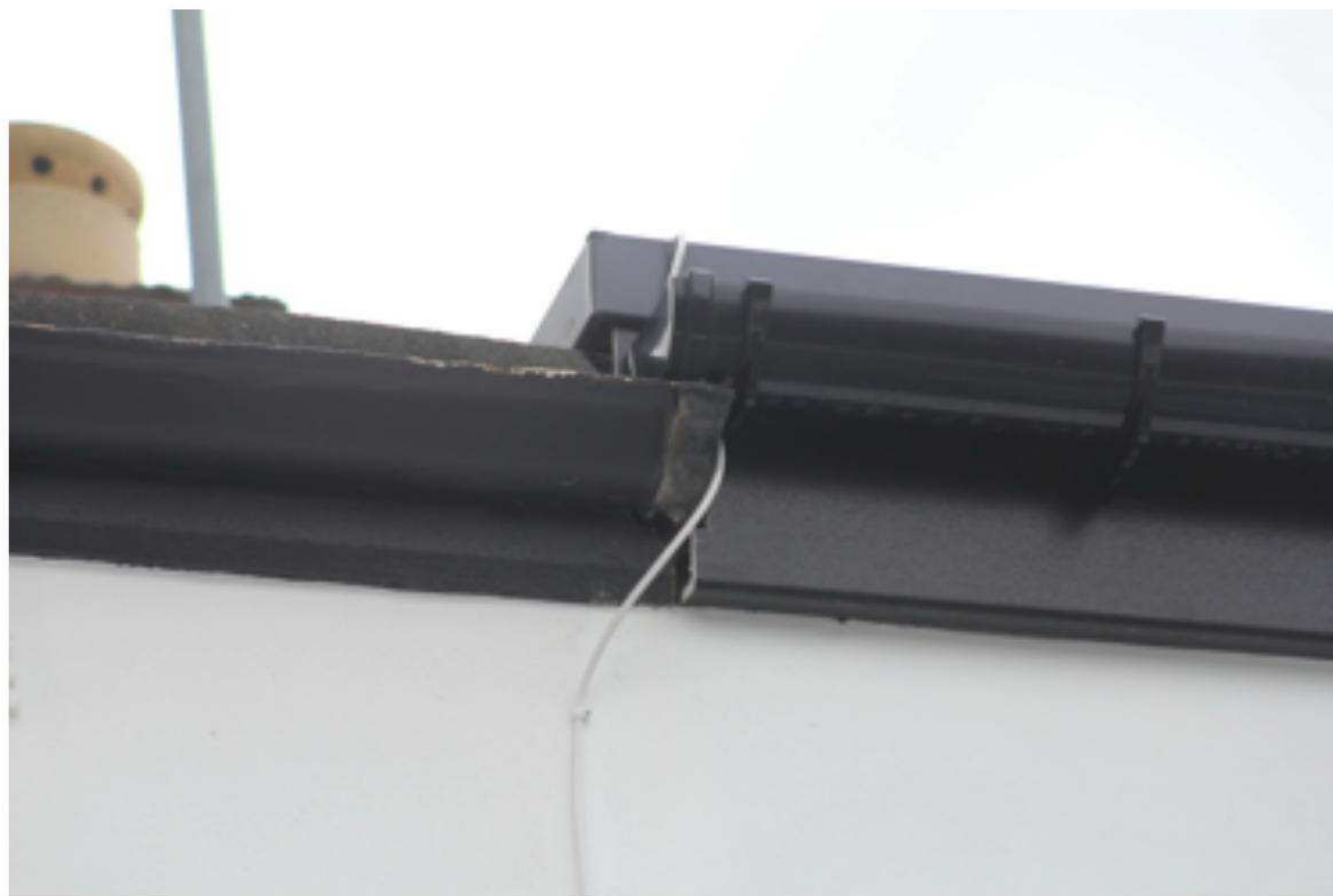
Figure 3: Changes to guttering between two properties
