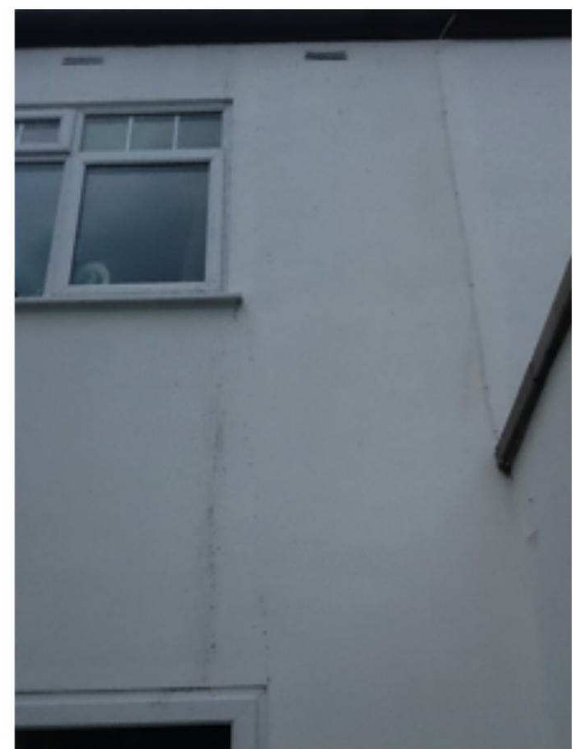
Figure 4: Dirt from guttering on wall
