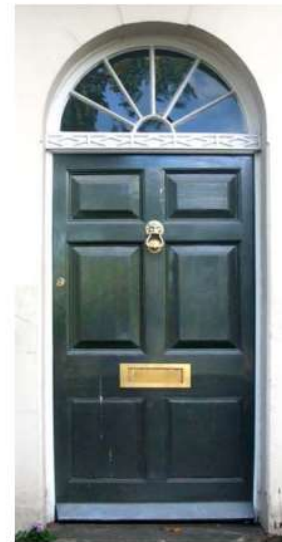
Fig.27 Correct Regency front door with the two bottom panels reeded but flush, the upper panels raised and fielded with a simple fanlight above, Montpellier Terrace
