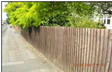
Figure 15 Poor wooden fencing on Hale's Road
